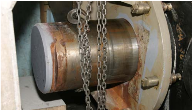
The existing shaft is removed in order to repair the hydraulic cylinder. Double sided gap in the mountings is discovered. Alternative corrective action is to replace both the cylinder mountings or replace the shaft with the Expander system.
